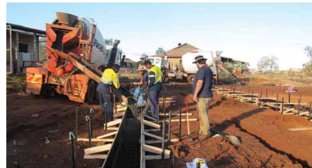
It's full steam ahead for several Gumala projects, including plans to construct approximately 150 homes for our Traditional Owners and their families over the next five years
