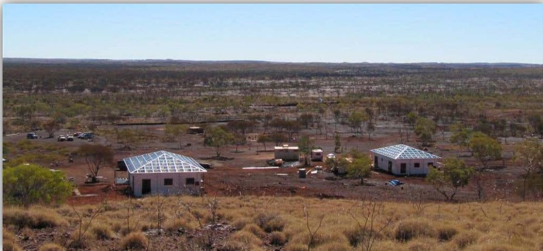
Houses currently being built at the Wirrillimarra Community, 150Kms east of Tom Price
